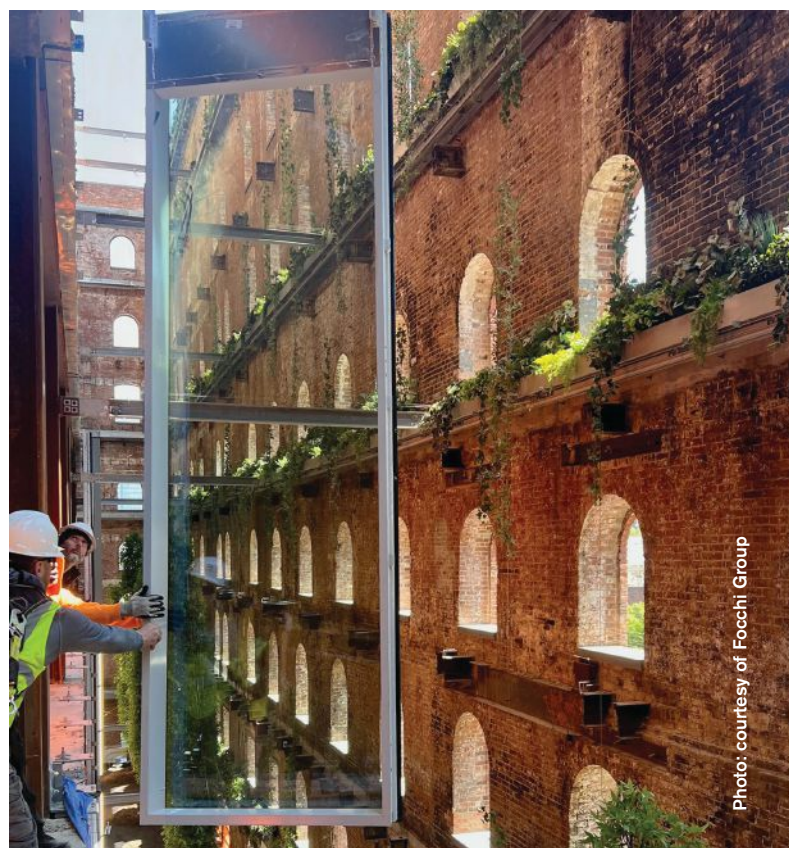
Focchi worked closely with Walsh Glass & Metal on the installation of the vertical as well as the curved panels.
