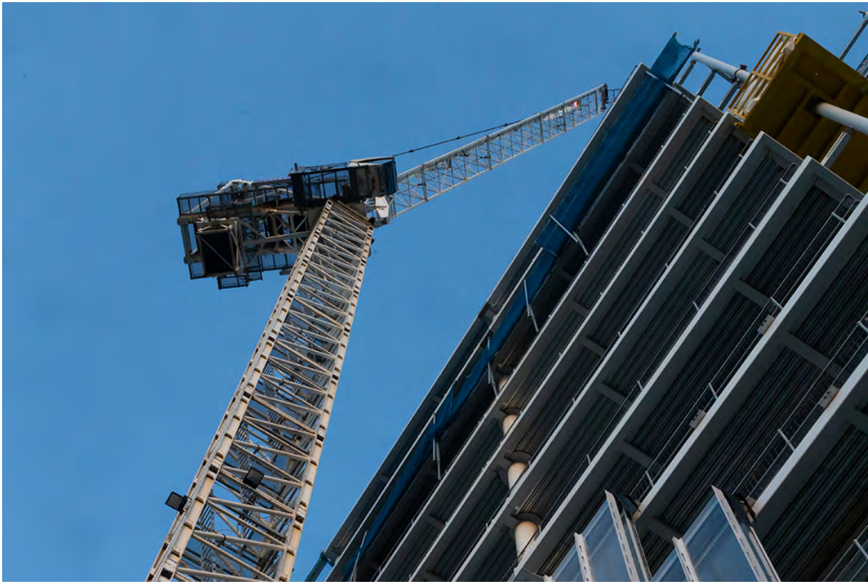
Steel was the only material considered for the bulk of the structural frame
